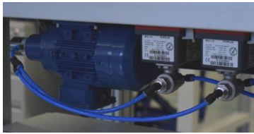
Controlled pump system
